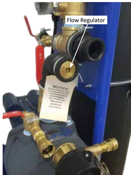
Figure 3: Flow regulator installed in 1-1/2" cam supply
