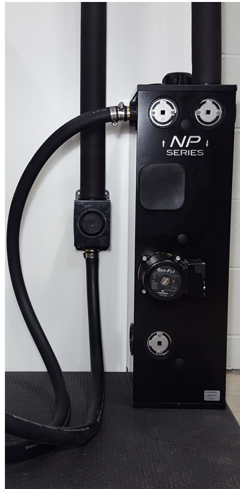
Figure 8: Wall mounted 3-way valve
